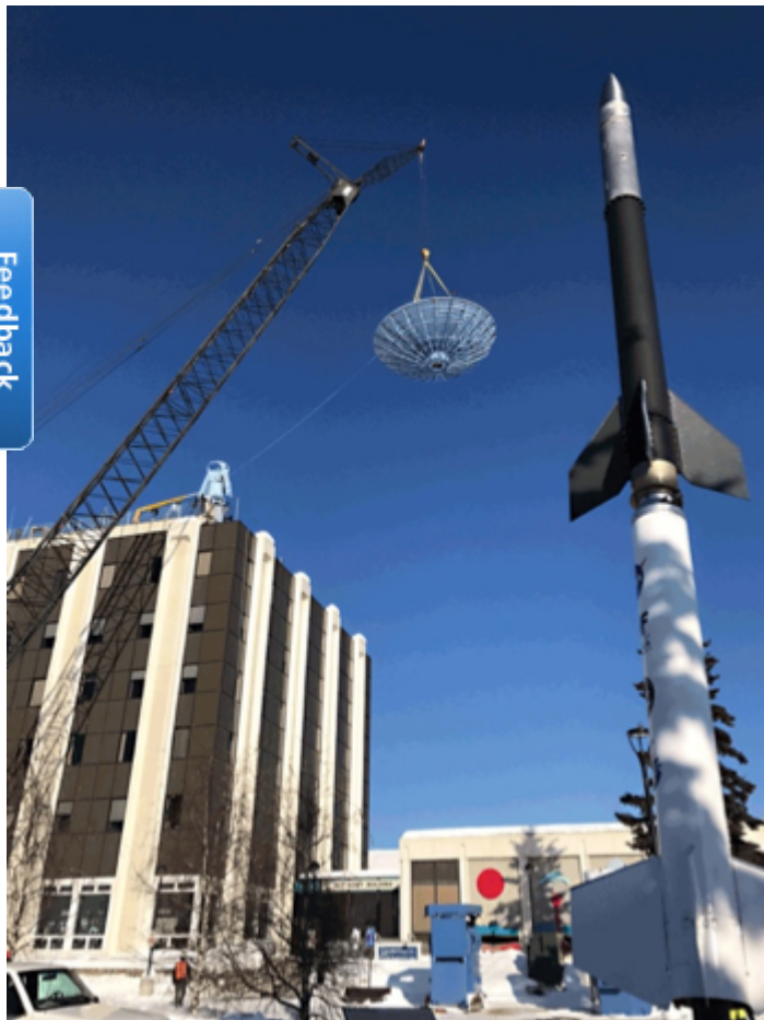
A 250-foot crane lifts the original antenna off the top of the Elvey Building, framed by an outdoor rocket display, part of the Geophysical Institute.
